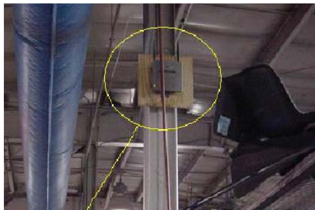
Figure 5-9 Access Point Mounted Directly to Steel Column
